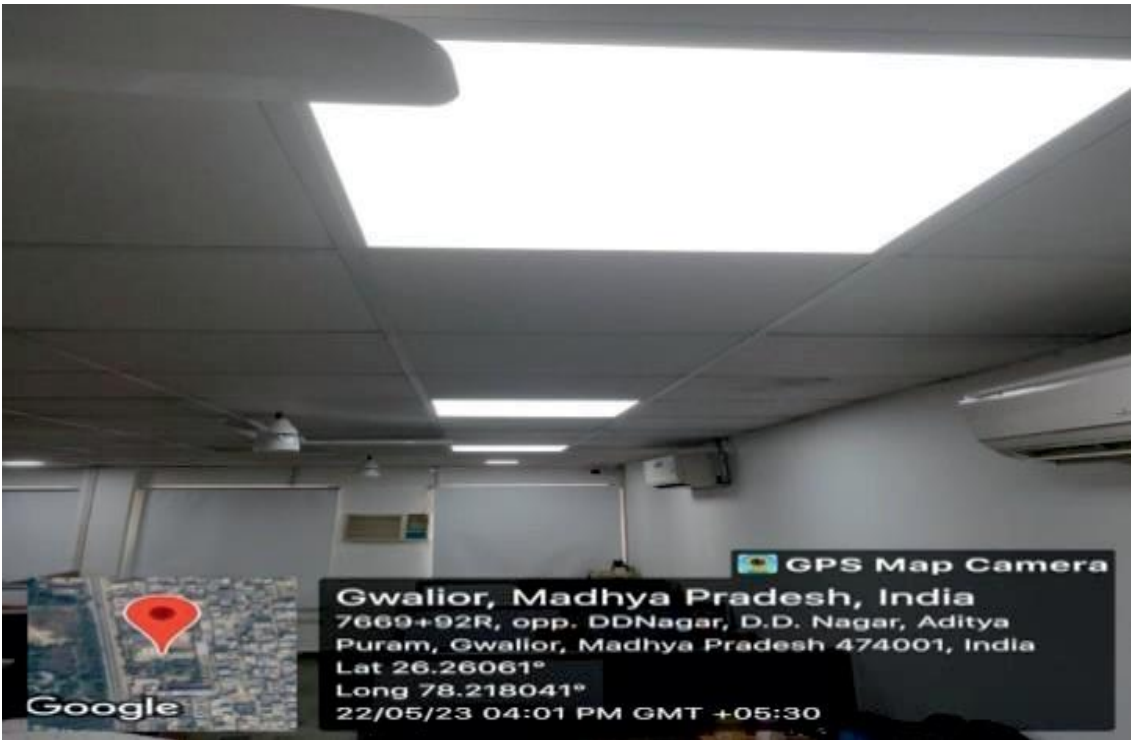
LED LIGHTS INTALLED IN FACULTY LOUNGE
